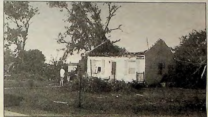
Pictured above is a home on the SW corner of Rt 18 and Chicago St. The roof was completely taken from this home with many trees uprooted.
