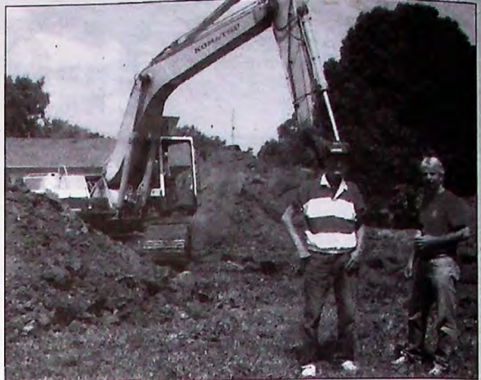
Pictured above L-R are Doug Ossola of J.W. Ossola construction sitting in his backhoe cab digging the basement for the new Habitat for Humanity house in Granville; Joe Panier, local Volunteer Manager and Mike Knapp, Building Chairman are overseeing the dig.
